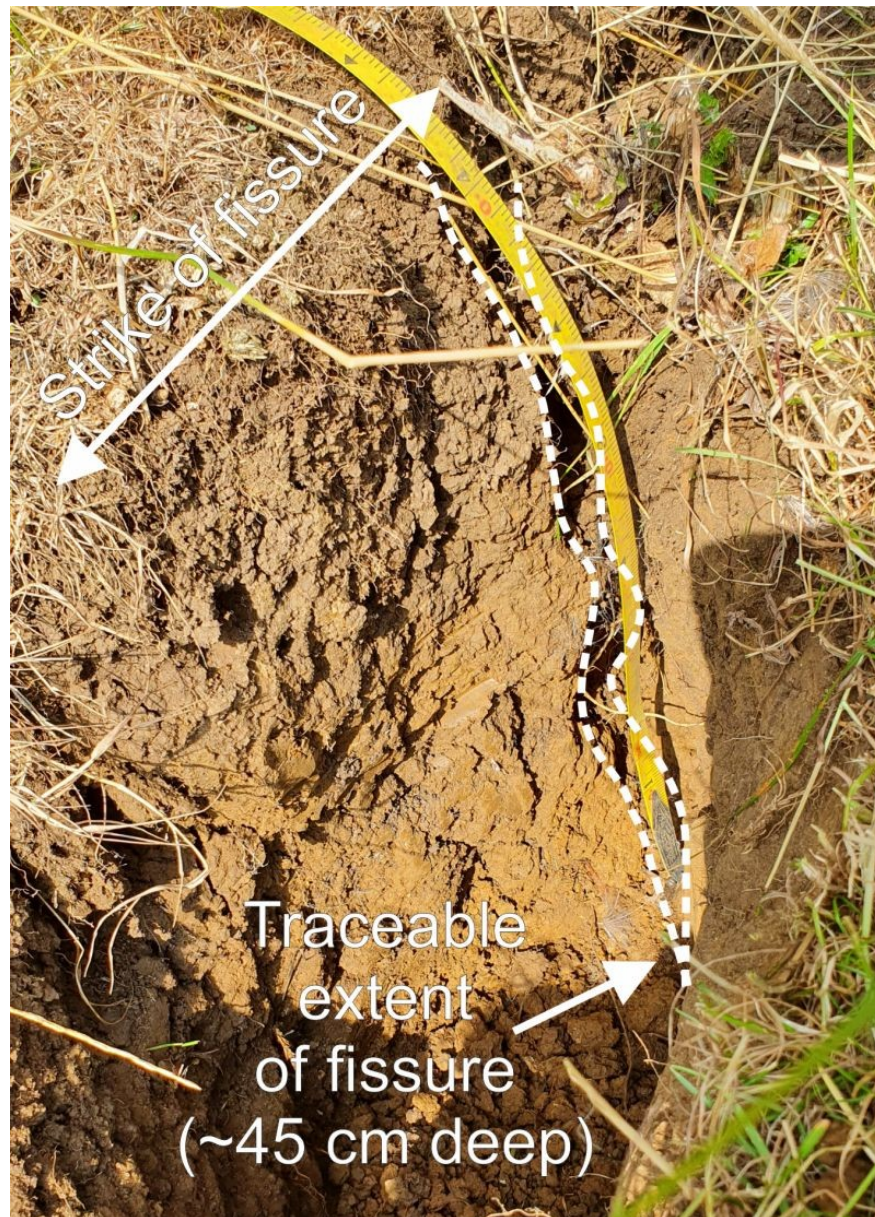
Figure S2: Example of desiccation-related fissuring observed at the Hollin Hill Landslide Observatory (HHLO). The photo shows a trench excavated into one of the larger surface fissures developed in the Whitby Mudstone Formation during an extended dry period. Moist soil was encountered from ~10 cm depth, while the
