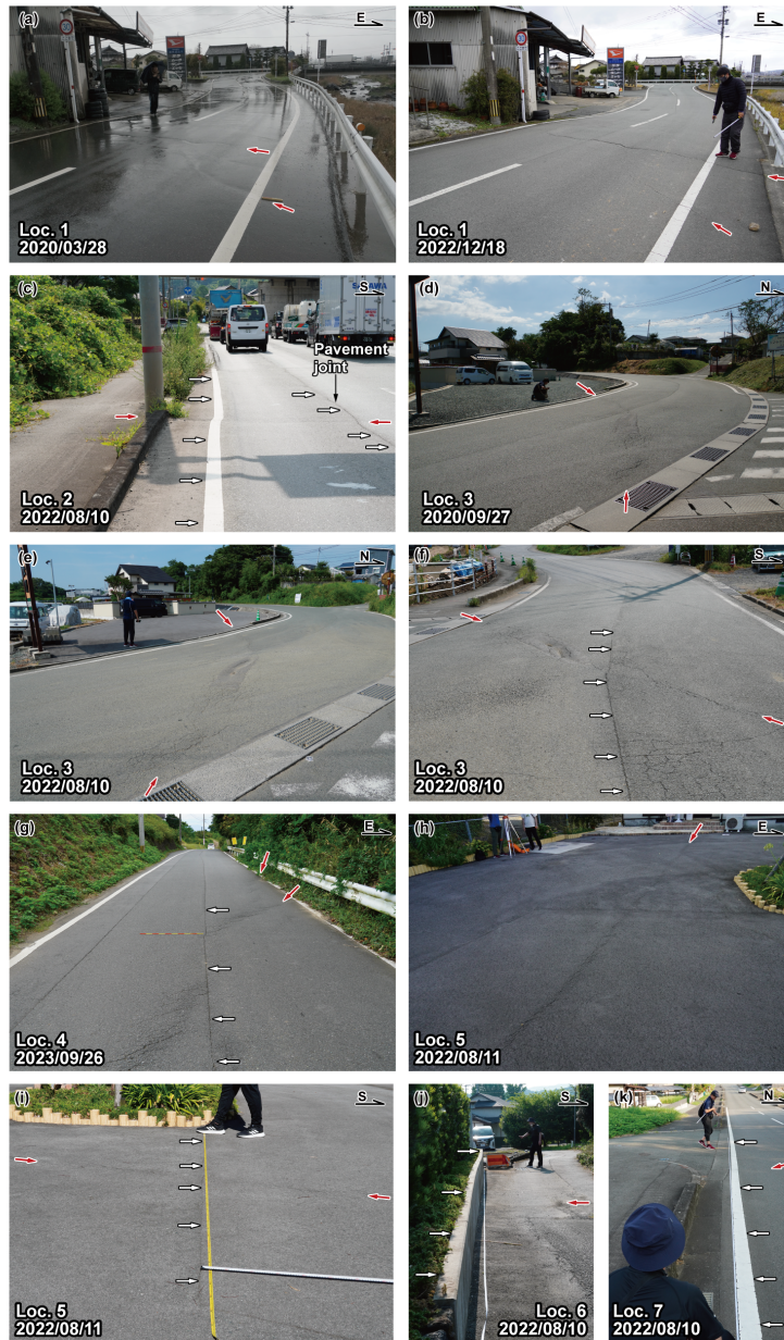
Figure 2 Photographs of the surface afterslip along the Hinagu fault. The locations are shown in Figure 1. Red arrows indicate the location of surface afterslips.
