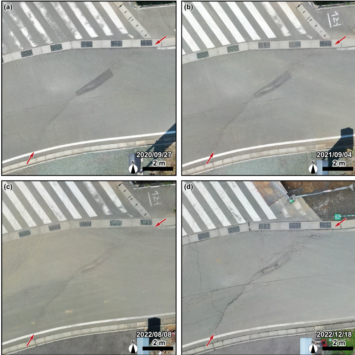
30 Figure S2. Temporal changes in the small graben-like depression at Loc. 3 in Takaki. Basemap is the orthographical image created using a drone image taken on 27 September 2020, 4 September 2021, 8 August 2022, and 18 December 2022, respectively. As time passes, the depression was growing to the northeast within the repaired patch of pavement. When we visited on 26 September 2023, the entire road surface had been completely repaired, and we were unable to observe the depression.
